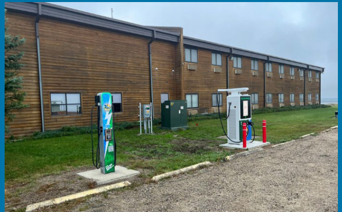
Figure 4. Level 2 and Level 3 Chargers at the Grand River Casino & Resort in South Dakota
